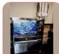
Purifier Water Tank
